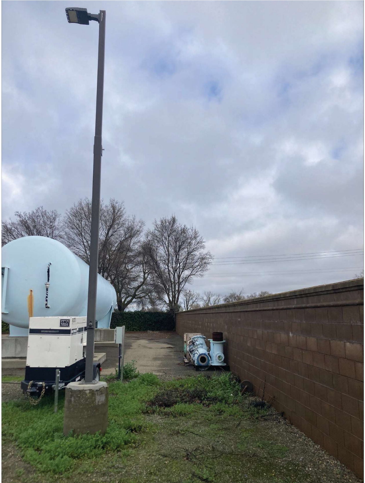
View of relative location of placement of 80' Tower (View facing North)
